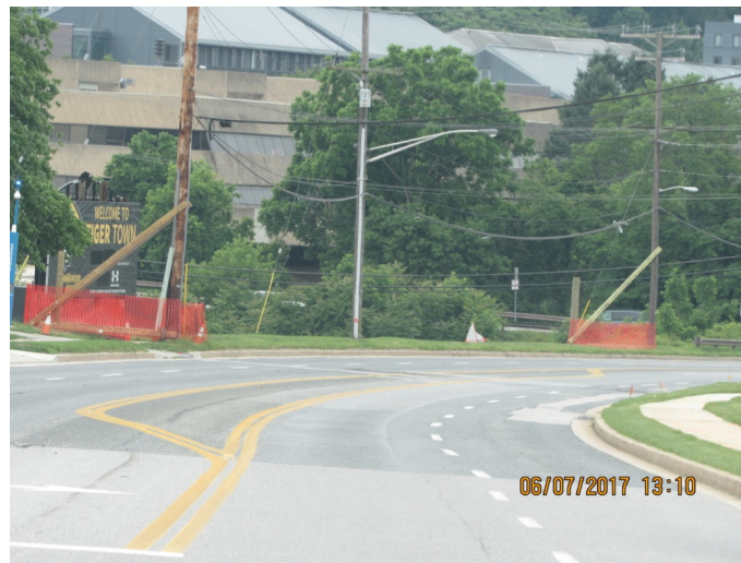
Utility poles are braced in advance of deep trench work for Towson Run Relief Sewer at the intersection of Osler and TTBlvd. 6/07/2017
